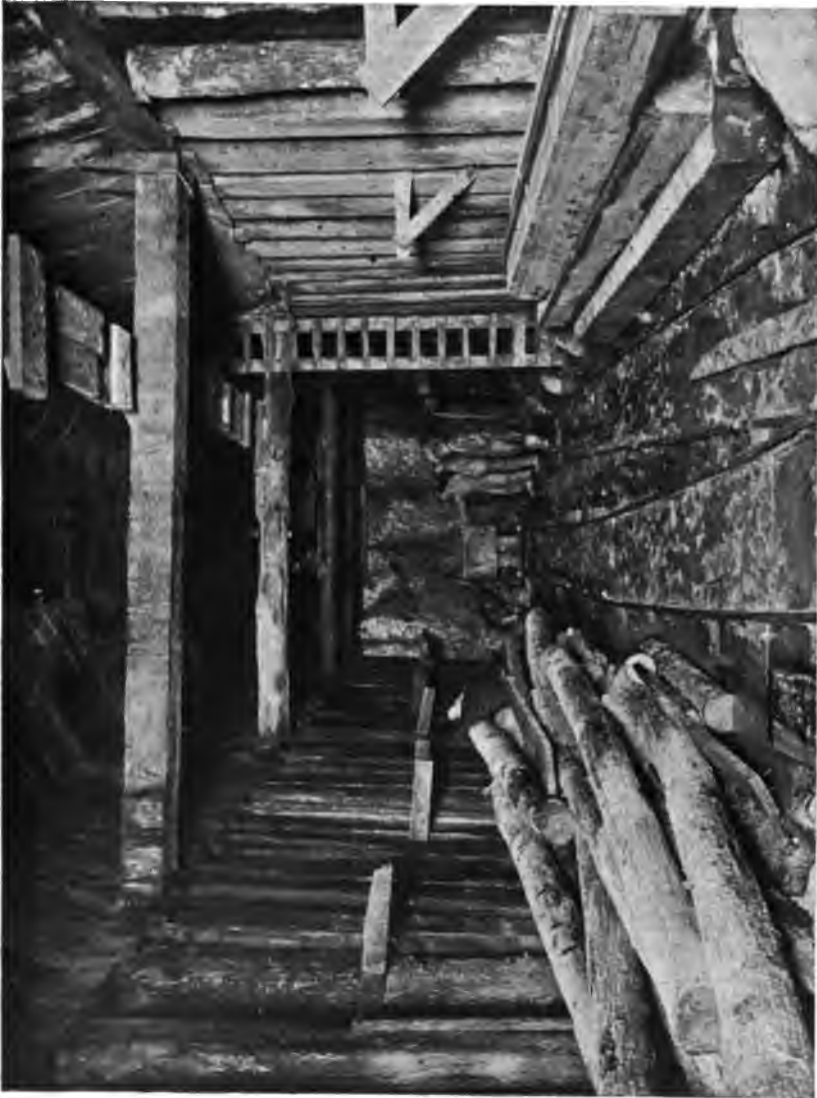
PLATE 146.—Contract 2. Garrison Tunnel. Timbering in heavy ground. Roof timbers “block to block” on account of heavy pressures.
